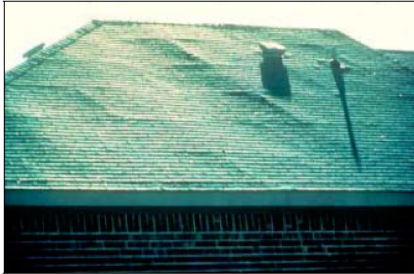
Degraded Plywood Sheathing from FRT Treatment Chemical and Solar Heating of Roof System
